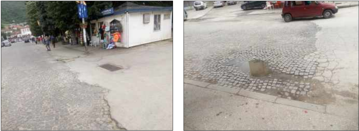
Fig.2 - Current state of the existing street and unformal parking lot across the square (bumpy and destroyed area)
